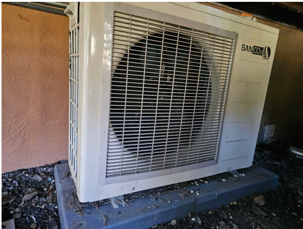
Heat pump for heating water, placed under deck (water tank in house where gas water heart was removed).
