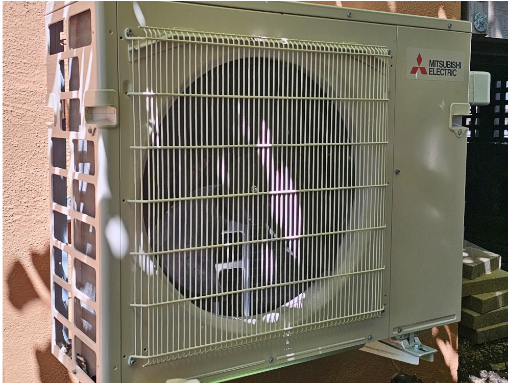
Heat pump for heating & cooling air, attached to side of house.
